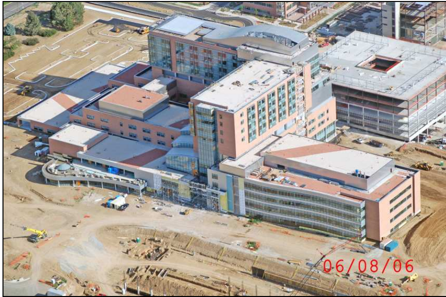
Aerial view of hospital and its main entrance with the outpatient wing to the right – June 2006
